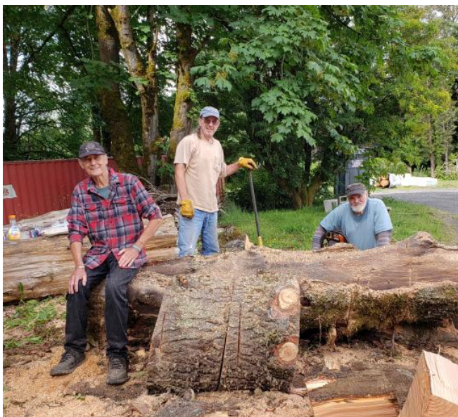
Volunteer woodcutters: Steve Lehl, Ken Smith, and Chuck Rollins help cut and clear fallen timber from the site.
